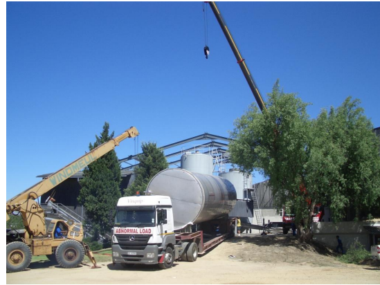
(b) In order to move the new tanks into the cellar, the roof had to be removed and various lifting and moving equipment was required.
